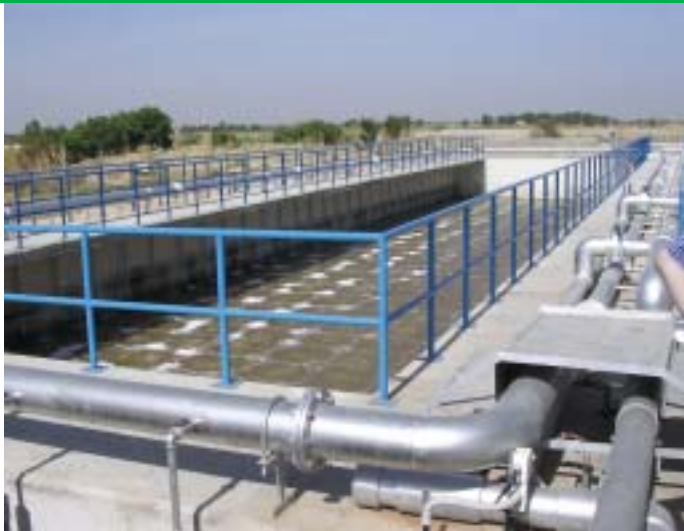
Wastewater treatment plant, Maiduguri, Nigeria
